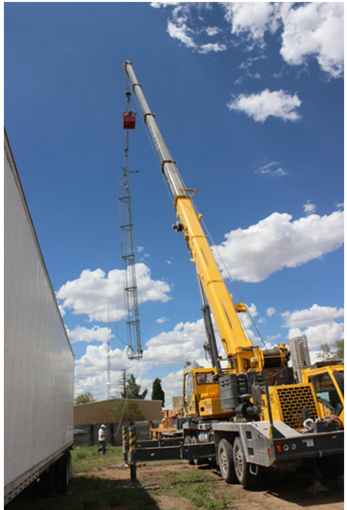
140 foot crane lifting the 70 foot tower (made from three Rohn 25 towers bolted together in a triangle – very heavy), swinging it to a vacant lot, and lowering to the ground.
